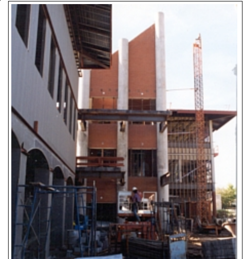
A view toward the elevator tower. The brick work has yet to be started on the main buildings.
