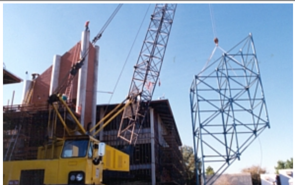
The last major piece of the building, the communication tower, is seen being hoisted to the top of the elevator tower.
