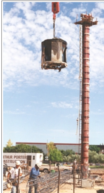
Construction started with the placement of the six columns that would frame the elevator and communication tower. This picture shows concrete being hoisted to the top of the steel mold of the first of the six columns.
