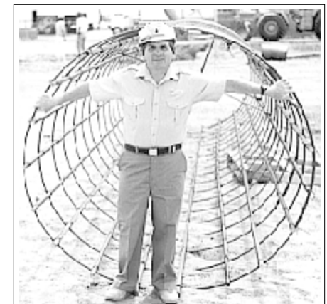
Chip Calamaio sizing up the rebar used in one of the six elevator columns.
