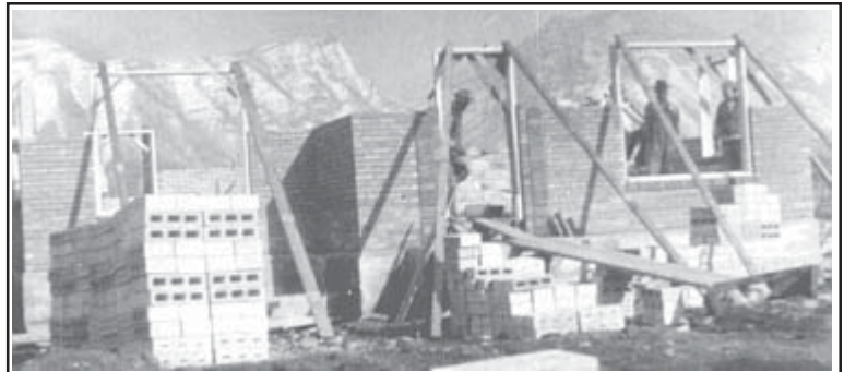
Construction began on our home in Orem in 1947 Three workmen are visible. One of them was probably Allen.
